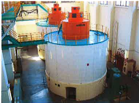
Figure 1 – Guthega Machine Hall
