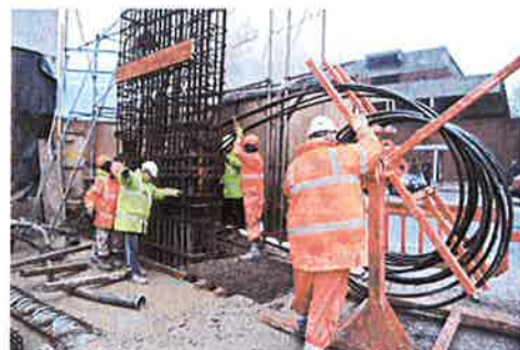
Figure 5: Ground loops in the reinforcing cage of a diaphragm wall during installation.
