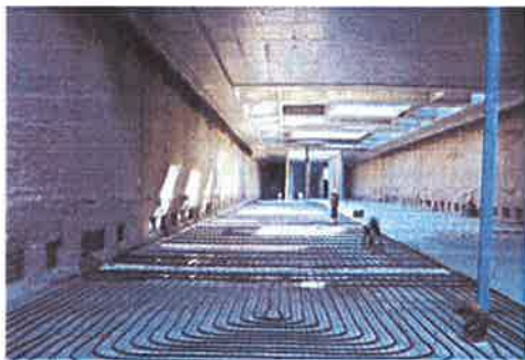
Figure 7: Horizontal ground loops in a mass concrete underground railway platform (Enercret, Vienna).
