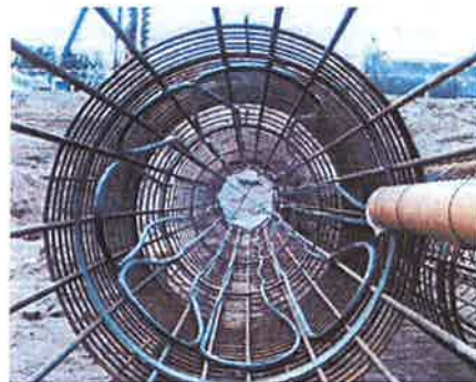
Figure 4: Ground loops in a reinforcing cage of a large diameter pile before installation (Enercret, Vienna).
